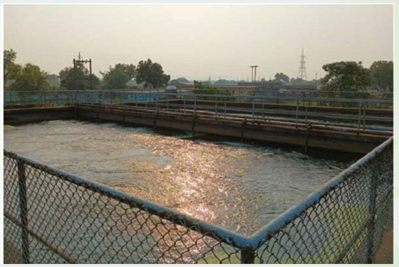
Water Reuse Plant
