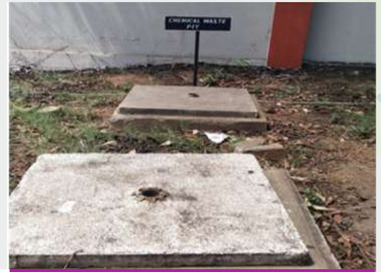
Chemical Waste Pit
