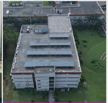
Roof and Façade Mounted Solar Panels
